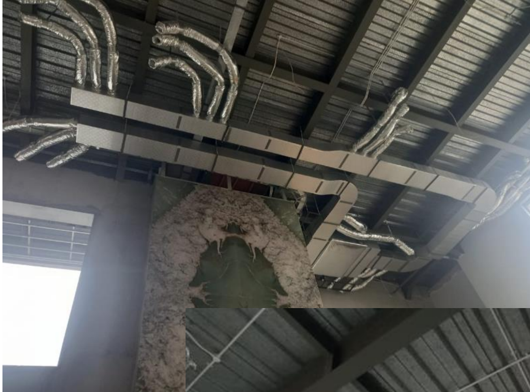
SUPPORT GANTUNGAN DUCTING DAN FLEXIBLE DUCT
